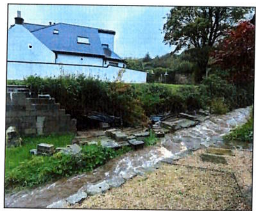
Figure 8 Wall down next to river.
